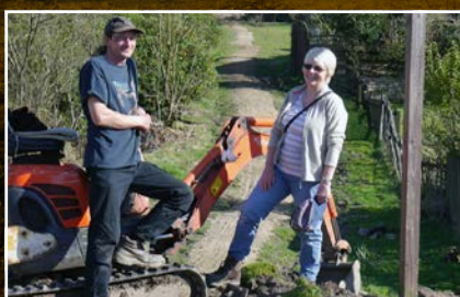
Helensburgh and District Access Trust Convener and Friends member, Anne Urquhart chats with the machineman as the path nears completion
