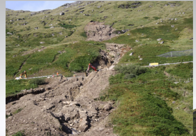
Transport Scotland says its proposed avalanche shelter will protect the A83 from debris flows – we are not so sure.
