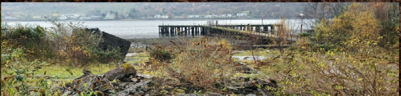
Dilapidated Arrochar Pier
